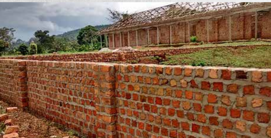
CONSTRUCTION IS NEARLY COMPLETE ON THE KKOBA COMMUNITY'S NEW SCHOOL. MATERIALS FOR THE SCHOOL WERE PURCHASED BY THE COMMUNITY USING PROFITS FROM THE PRODUCE TRADING BUSINESS STARTED WITH FUNDING BY THE KAIN FOUNDATION
